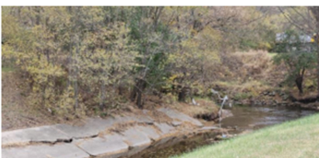
Figure 2: Concrete channel discharging into North Fork of Kent Creek. Broken concrete and debris are present.
