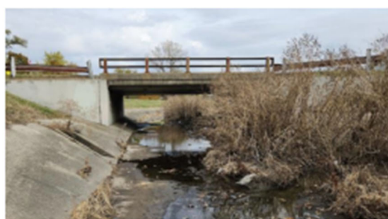
Figure 3: Concrete channel passing under Gilbert Avenue. Invasive brush impedes flow.
