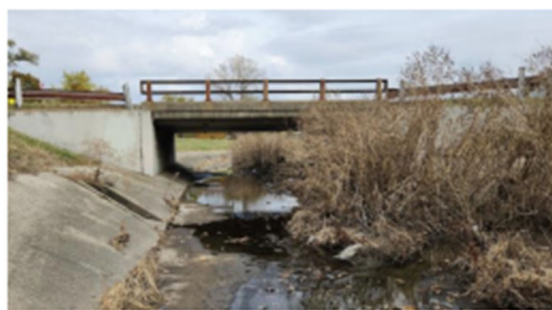
Figure 3: Concrete channel passing under Gilbert Avenue. Invasive brush impedes flow.
